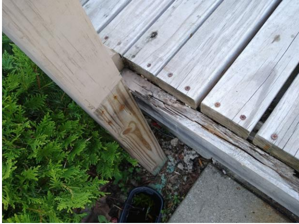
2013 deck that rotted
