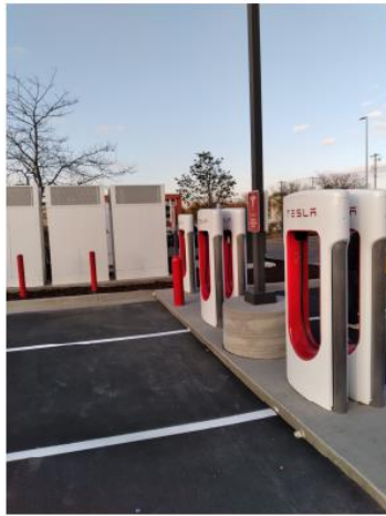
Charging Cabinets and Charge Posts
