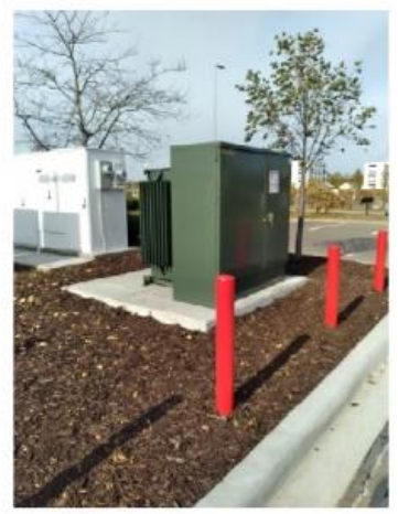
Switchgear and Transformer
