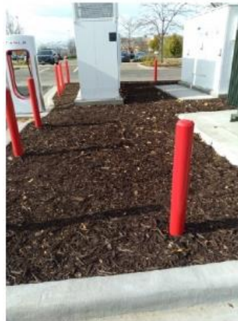
Cabinets and Switchgear
