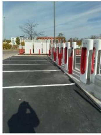
Charging Cabinets and Charging Posts
