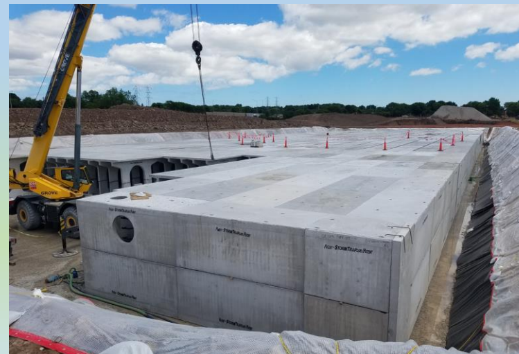
Underground Retention Basin
